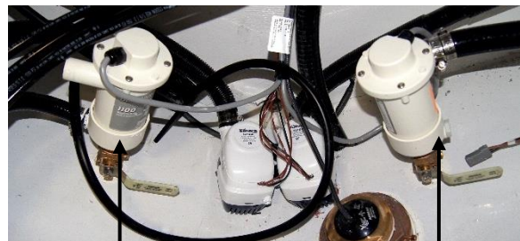
Pumps To Fill Valves
