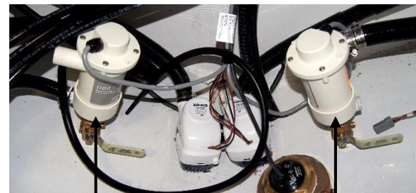
Pumps To Fill Valves
