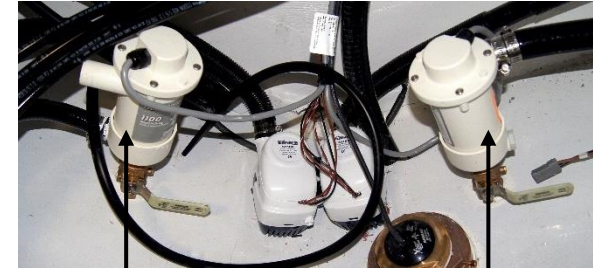
Pumps To Fill Valves
