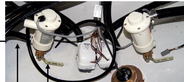
Shut Off Valve
