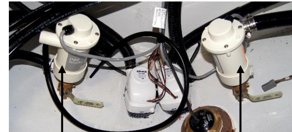
Pumps To Fill Valves
