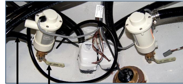
Shut Off Valve
