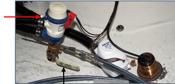
Pump To Fill Valves
