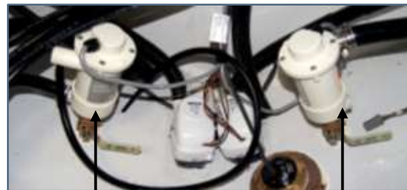
Pumps To Fill Valves
