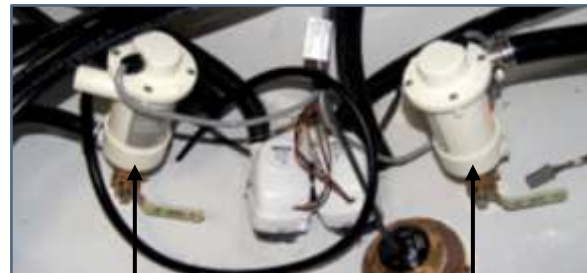
Pumps To Fill Valves
