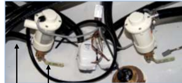
Shut Off Valve
