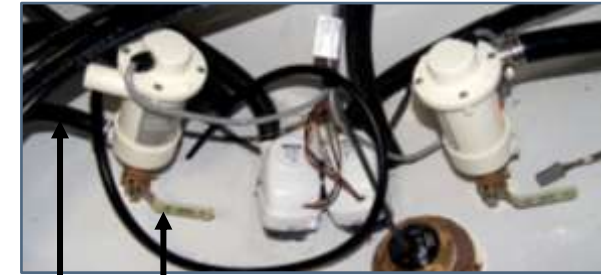
Shut Off Valve
