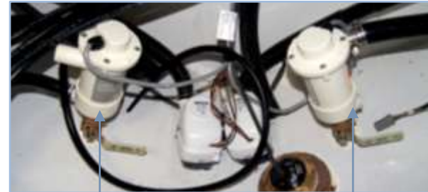
Pumps To Fill Valves
