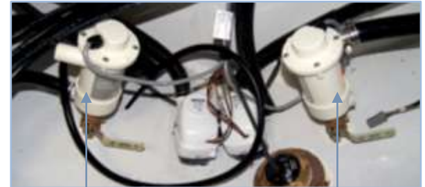
Pumps To Fill Valves
