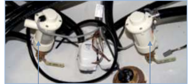
Pumps To Fill Valves
