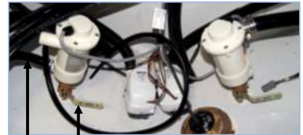
Shut Off Valve
