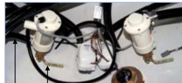
Shut Off Valve
