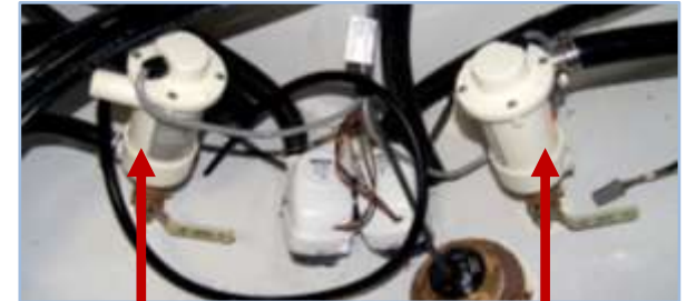
Pumps To Fill Valves
