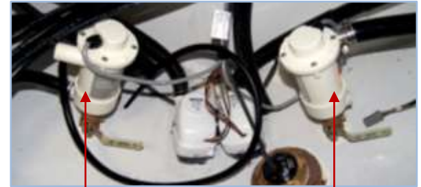
Pumps To Fill Valves
