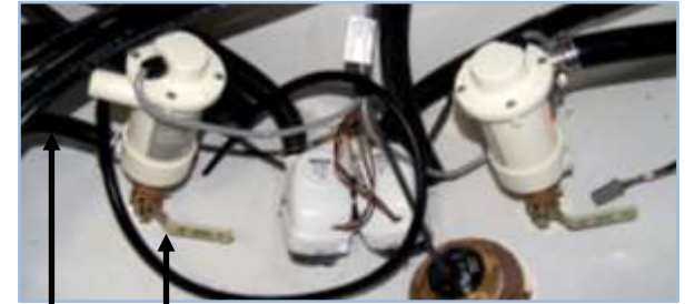
Shut Off Valve
