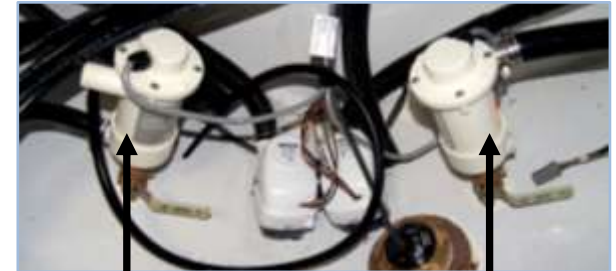
Pumps To Fill Valves
