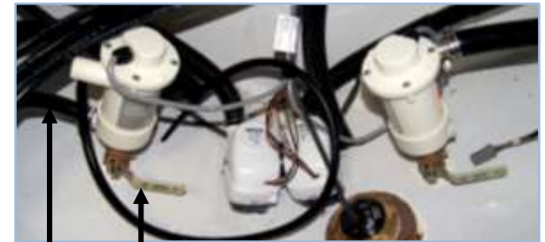
Shut Off Valve
