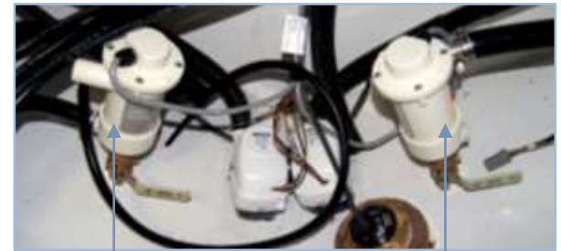
Pumps To Fill Valves
