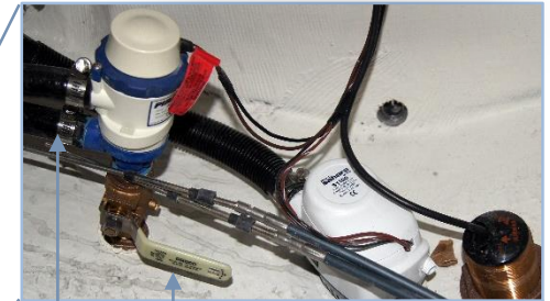
Shut Off Valve
