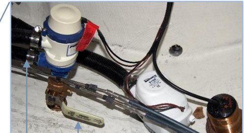
Shut Off Valve
