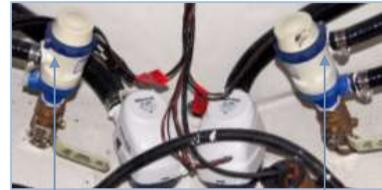
Pumps To Fill Valves
