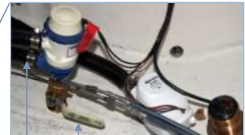
Shut Off Valve
