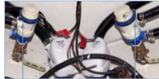
Pumps To Fill Valves
