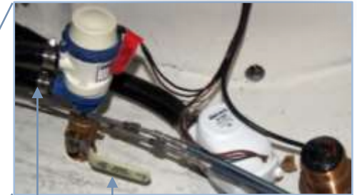
Shut Off Valve
