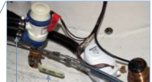
Shut Off Valve
