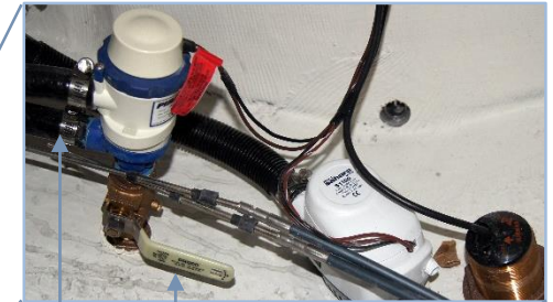
Shut Off Valve
